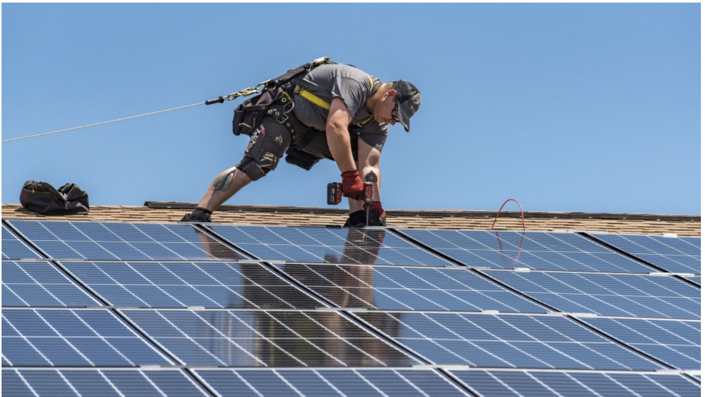
Installing solar PV panels on a home in the Dover Air Force Base in Delaware. Credit: Roland Balik, U.S. Air Force.
